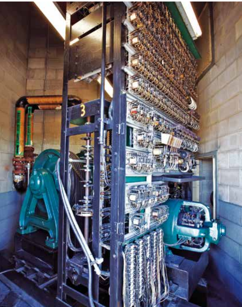
An outdated system equipment room.
